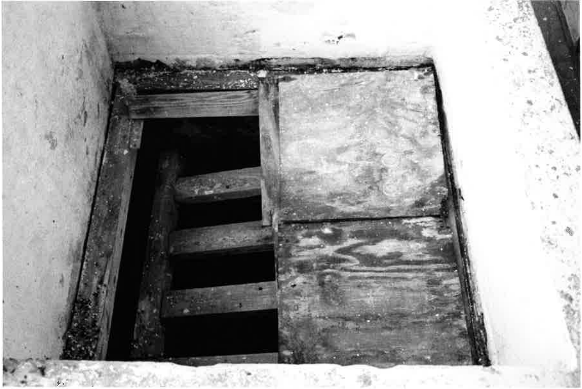
Figure 34: Wooden Grate Covering Shaft outside Chapel Door to Male Slave Dungeon, Cape Coast Castle
